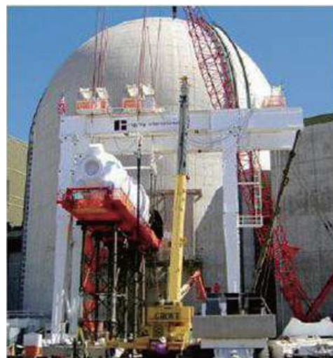
Steam generator on transporter
