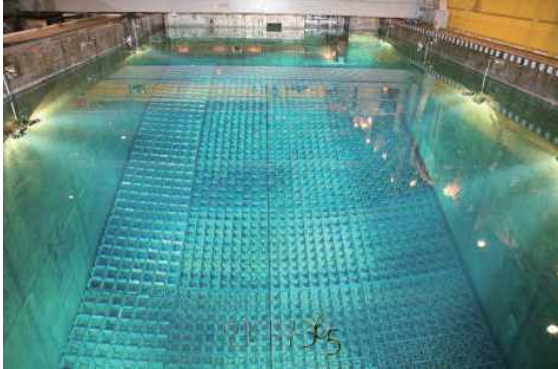
저장조 (storage pool)
